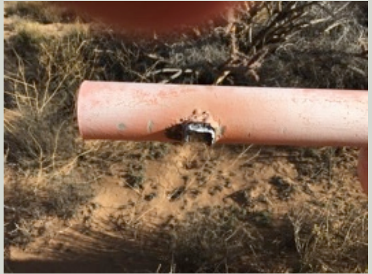
Lock Bolt broken from gate
